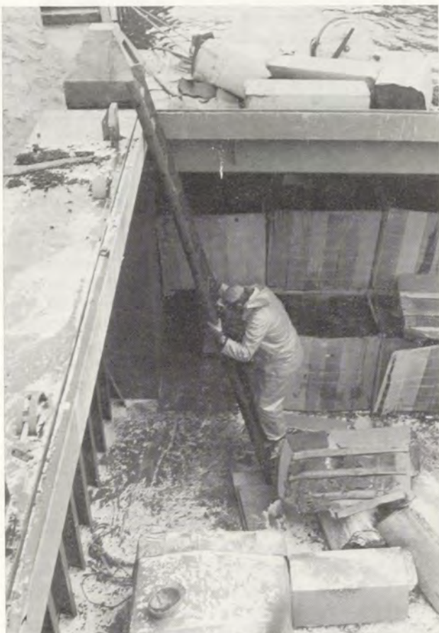
Figure 26 - Accessibility of the barge hold must be improved.
